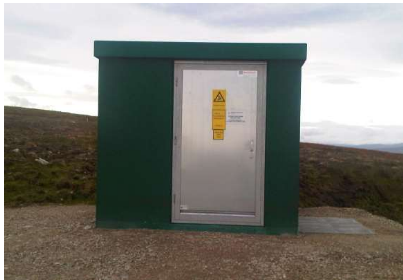
Figure 6.1: Typical Transformer Housing
